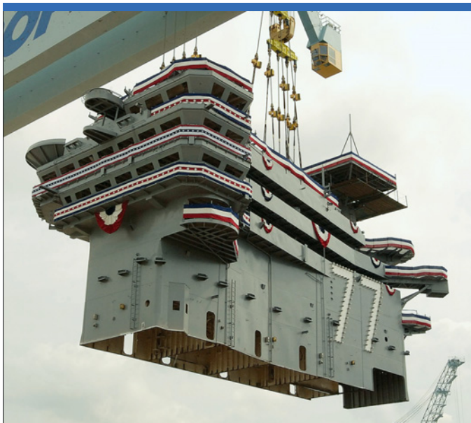
The 700-tonne 'island' as it was being carried onto the last of the Nimitz class carriers, the USS George H.W. Bush, on 8 July 2006. (Newport News)
